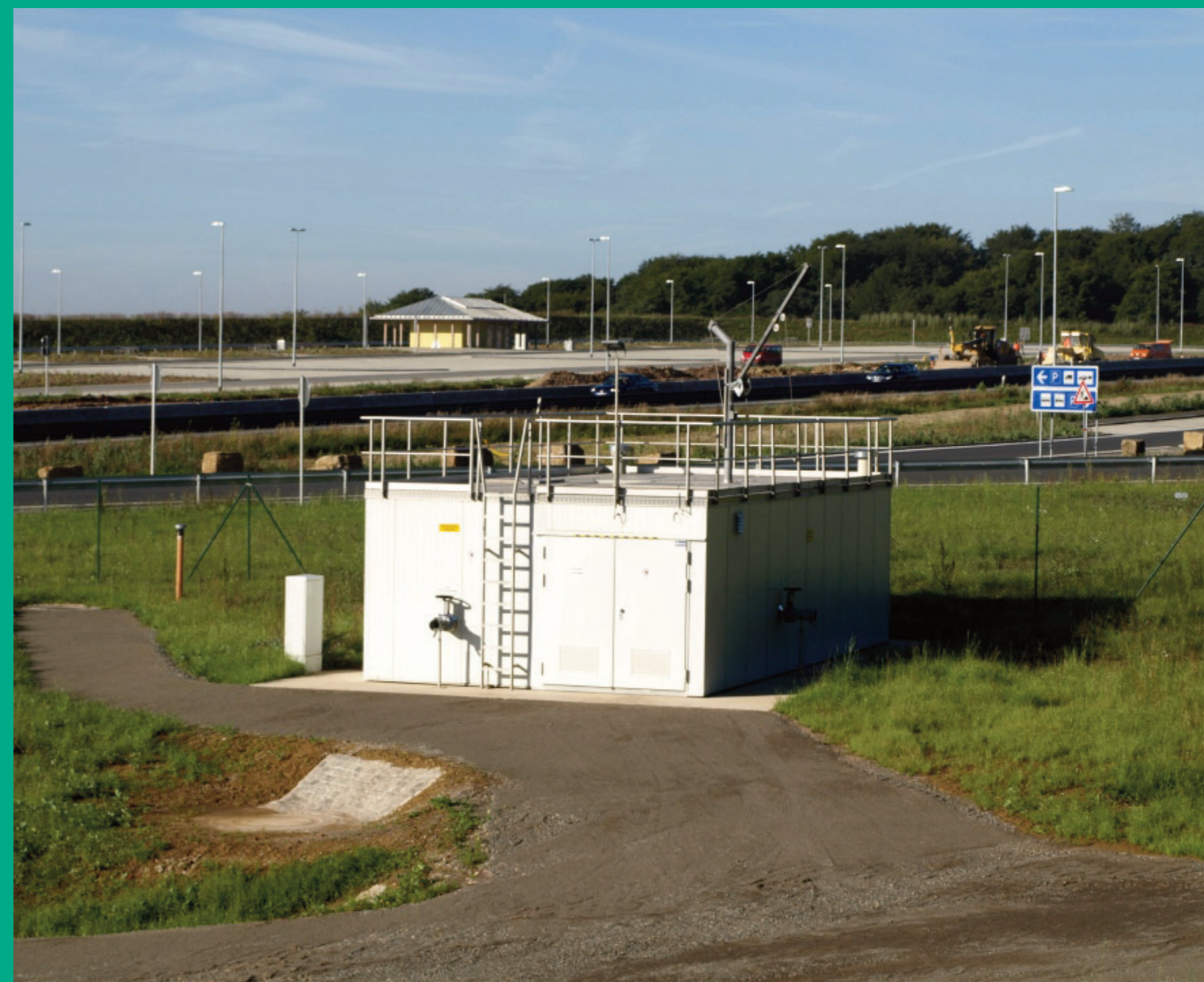
PWC Plant of Martin Systems on the A3
