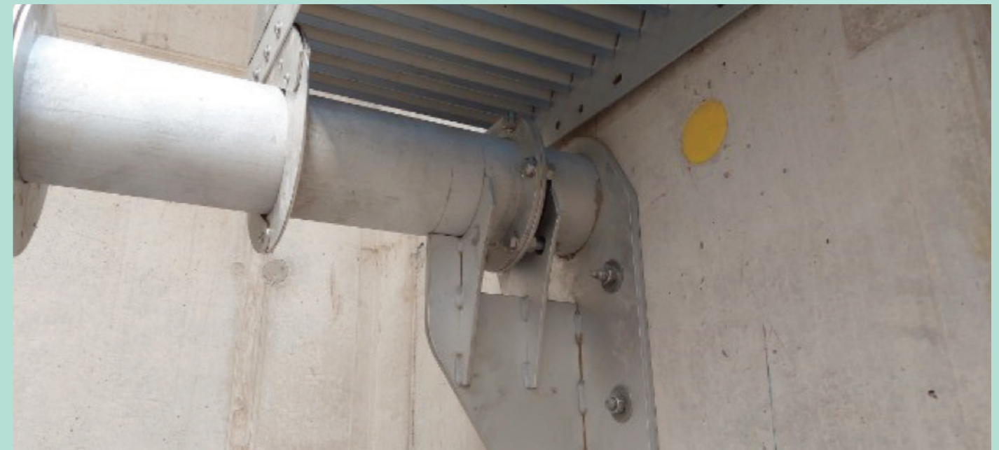
Bearing for inclined clarifier modules in a stormwater tank for the K20 section of the BAB7 in Hamburg
