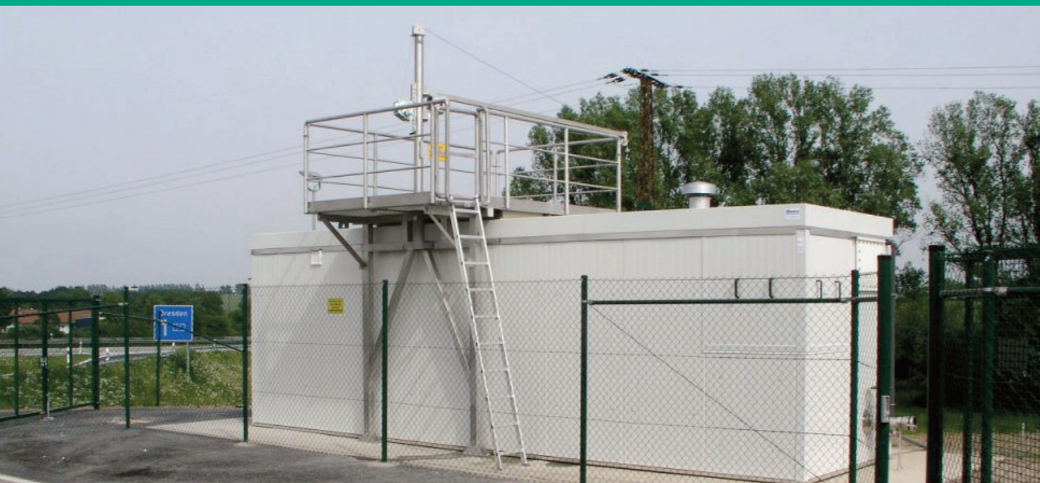
PWC Plant of Martin Systems on the A72
