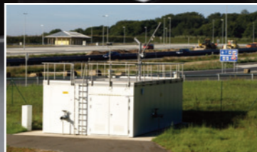
Wastewater treatment plant for highway service area
