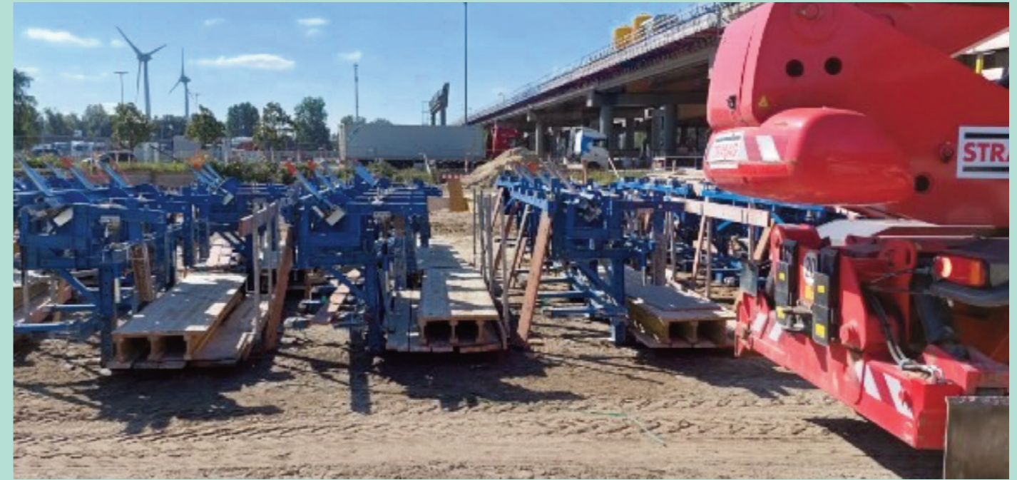
Sedimentation surface on a site on the K20 section of the BAB7 in Hamburg
