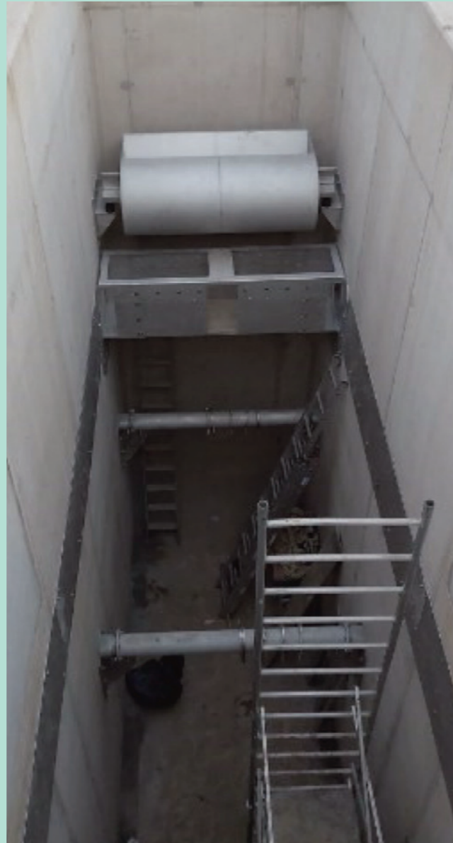
View into the sedimentation chamber of a stormwater clarification tank for the K20 section of the BAB7 in Hamburg (before fitting the inclined clarifier module). In the background: tipping bucket for cleaning the base of the stormwater clarification tank
